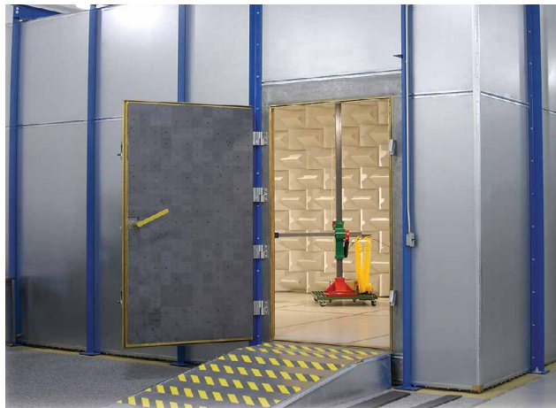
FIGURE 3. A chamber without a pit requires an equipment ramp. A swinging door lined only with ferrite tiles will clear the door opening. Courtesy of Panashield.
