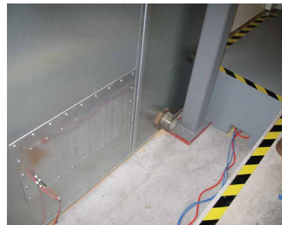
FIGURE 4. A penetration panel sits below the building floor, providing access to cables that run under the chamber's raised floor. A pipe opening alongside the panel provides access for additional cables and hoses.
